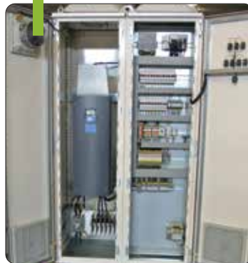
Winch control cabinet with frequency converter
