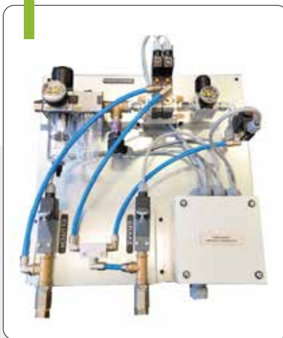
Winch pneumatic control panel
