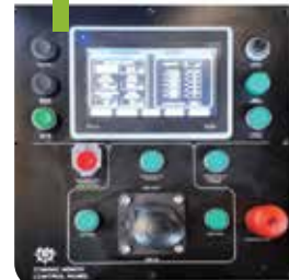
Towing winch control panel with display unit.
